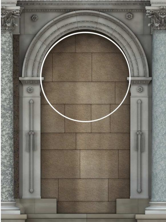
Figure 14. The arch above the third niche (from the left). The deviation from perfect circularity is clear.
